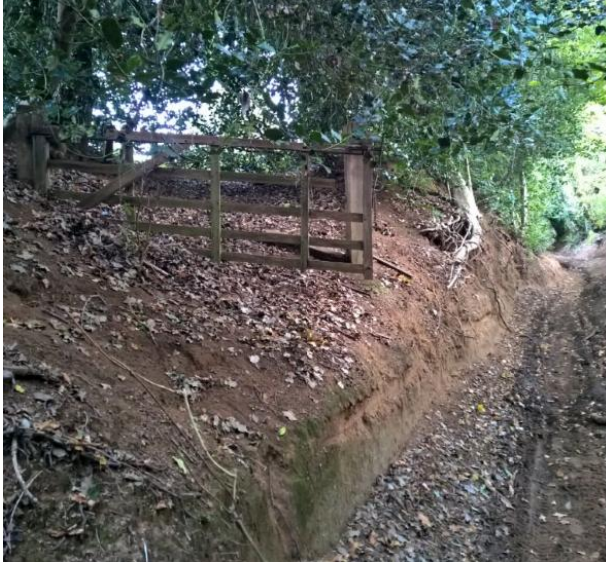
The sunken nature of the track and the rapid erosion of the sand are clearly shown here by this 'hanging gate' on Ride Lane
